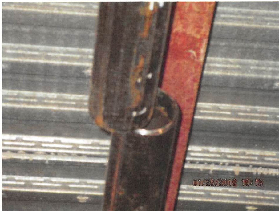
Figure 6 - Image attached to the January 26 email showing installed but uncapped pipe. DX548 at LEEB_000286748. Dickerson described this as “either chiller piping or gas piping hung in the air that is not capped on the ends,” an issue that “was specifically discussed.” Tr. at 1310. When pipes are unsealed “air or humidity or moisture” can get inside the pipe, which can cause the inside of the pipe to rust. Tr. at 1312.
