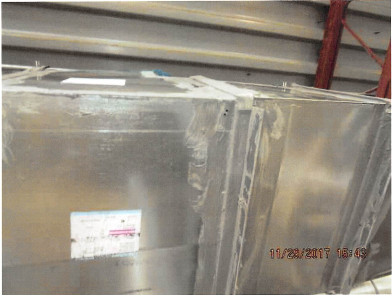
Figure 3 - One of the images attached to the November 29 email depicting installed ductwork with two small holes in it. DX841 at LEEB_000360282.
