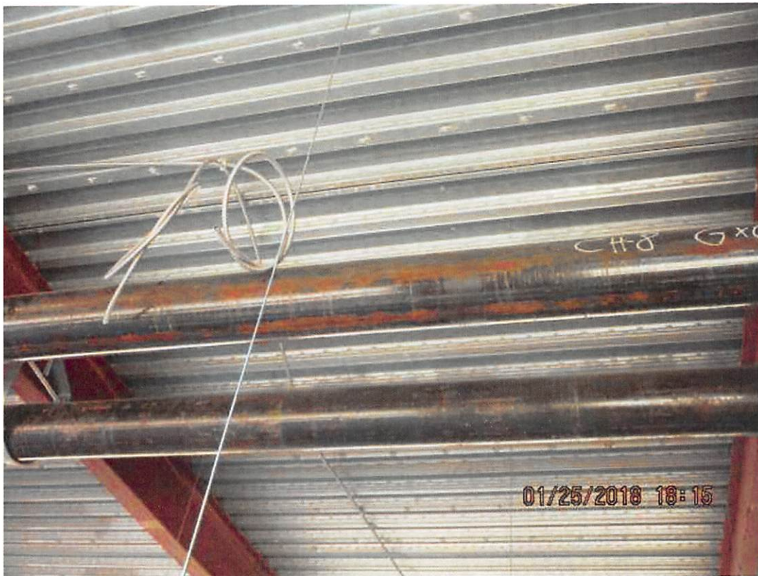
Figure 4 - Image attached to the January 26 email showing rusted pipe. DX548 at LEEB_000286736.
