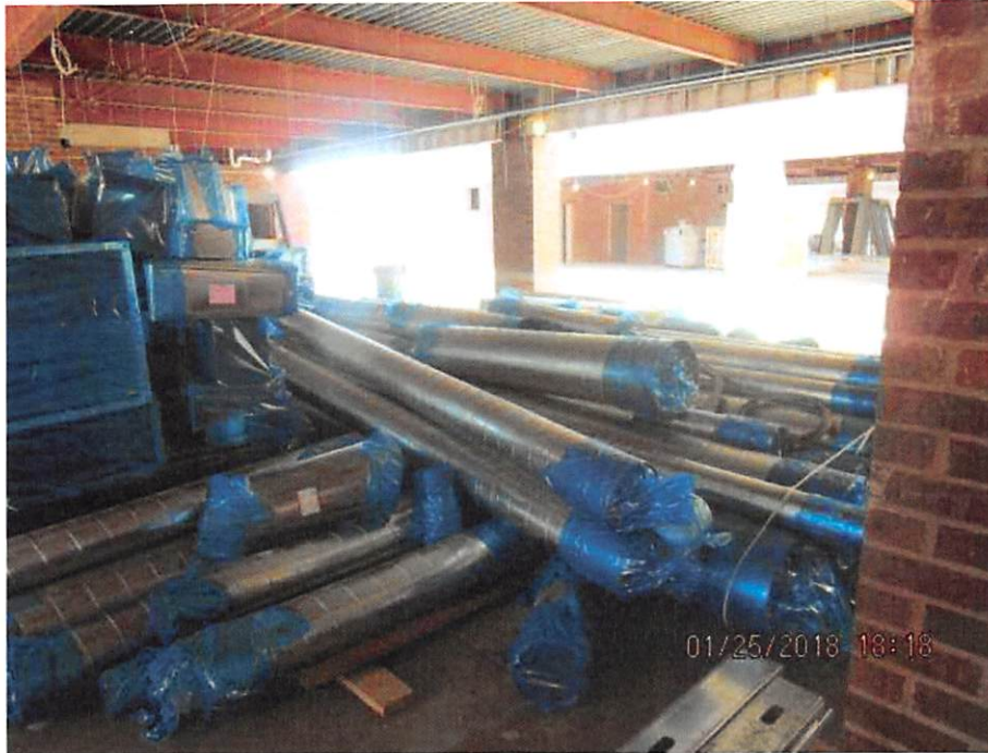
Figure 5 - Image attached to the January 26 email showing haphazardly stacked ductwork. DX548 at LEEB_000286745. As Dickerson explained, “[a] lot of this ductwork had dents in it, and when we install the ductwork, you can’t have large dents in it, and this was just not . . . stored in a manner that will protect it.” Tr. at 1309. The court agrees.
