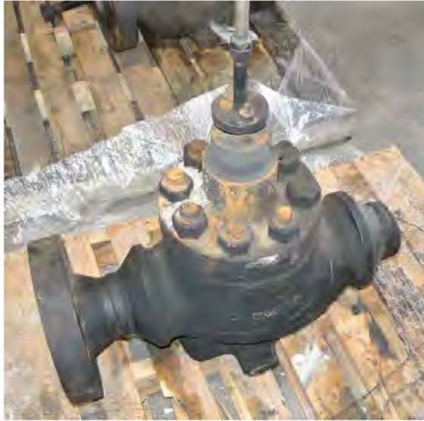
Image of FV-241 after it fractured. The right-hand side of the valve is missing its flange.
