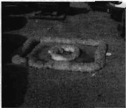
Properly Protected Drain Inlet
