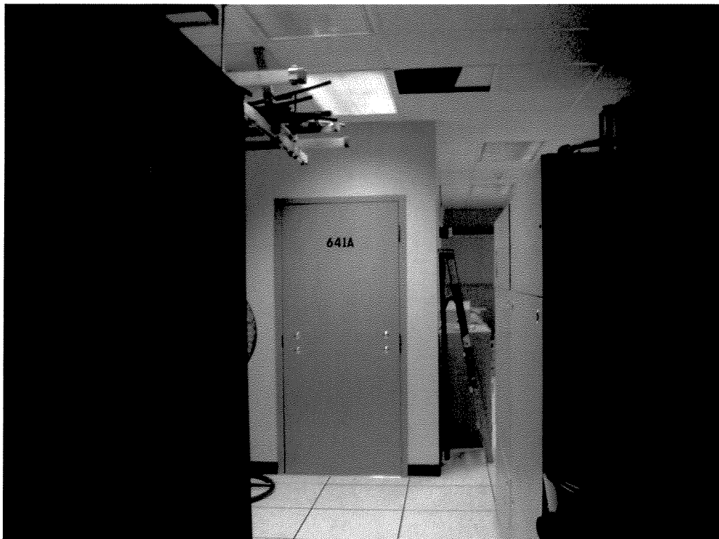
Entrances to the “secret room” at AT&T central office, 611 Folsom St., San Francisco
