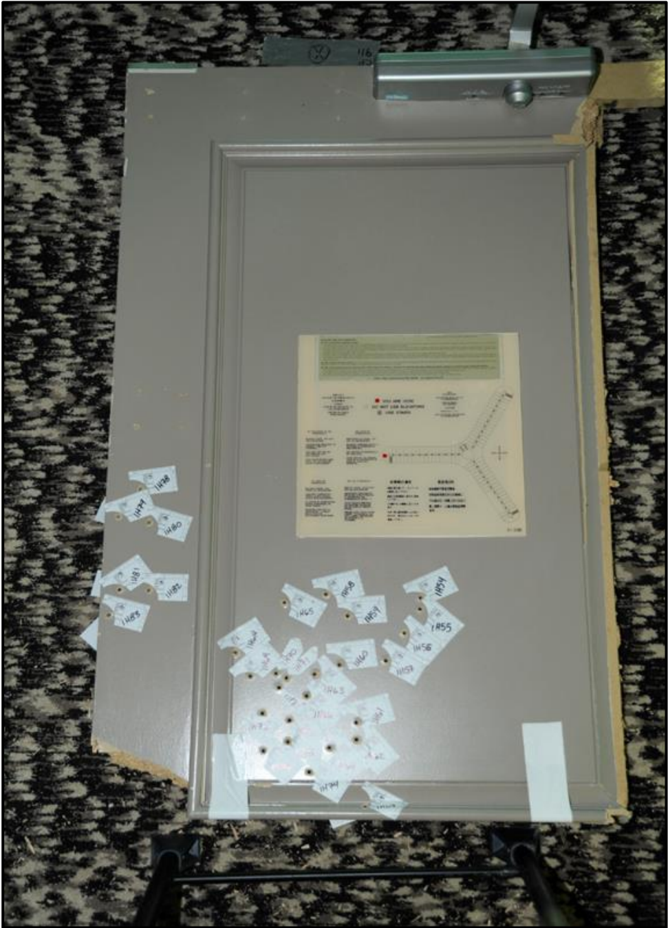
(Damage to entry door of room 32-135)
