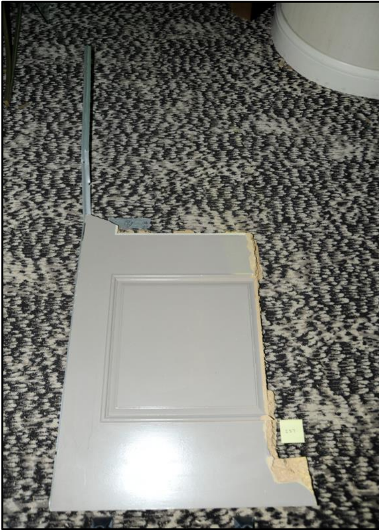
(Damage to entry door of room 32-135)
