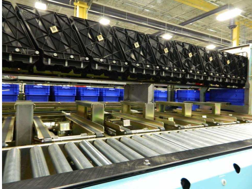
Defs.' Mot. Ex. 10 (photograph of rails, blue plastic bins, and conveyor buckets).
