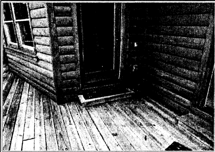
Right Front Exterior Door Weather
