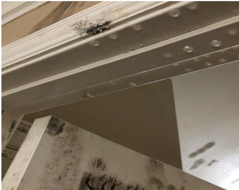
Figure 2 Moisture and Mold Damage [58-6 at 13]
