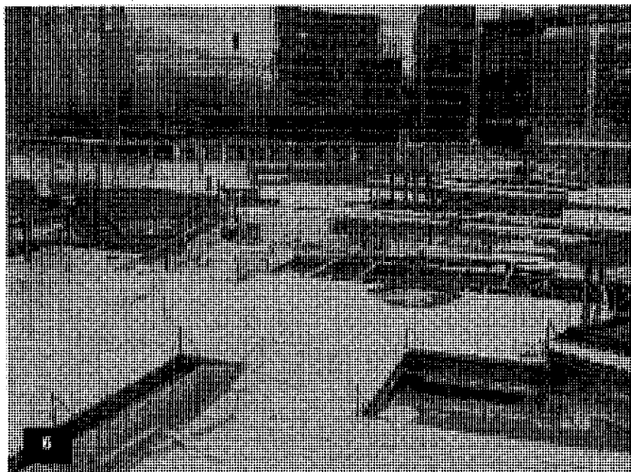
Podium Pool Deck – View of the structural steel framing and metal decking with pool, spa and escalator openings framed.
