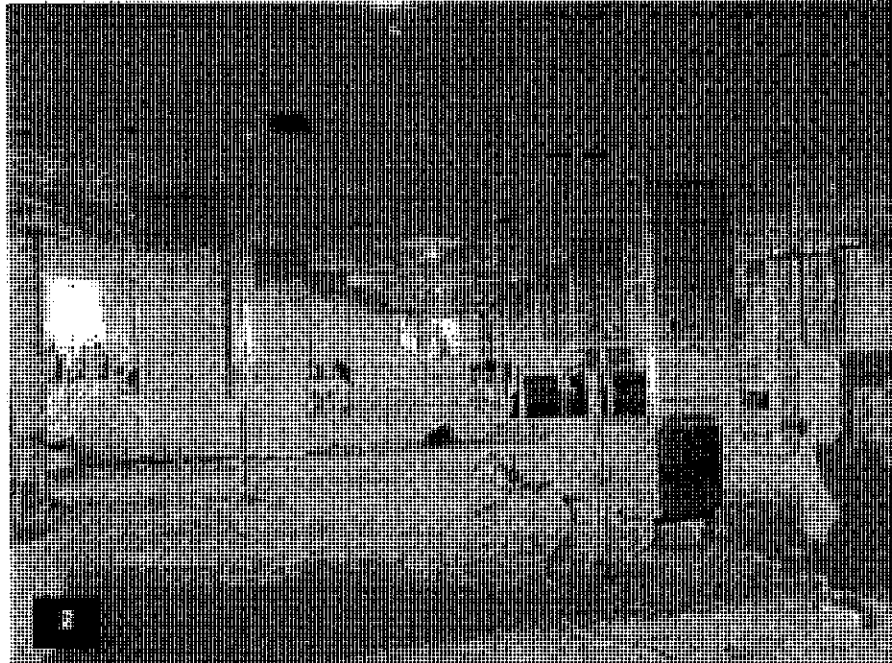
Tower Level T66 - View of the following in process items: domestic hot and cold water supply lines and vertical mechanical duct.
