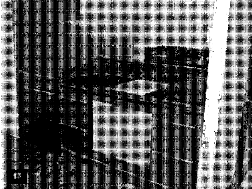
Tower Level T2 – View of a completed typical condominium kitchen completed excluding the cooktop and oven.
