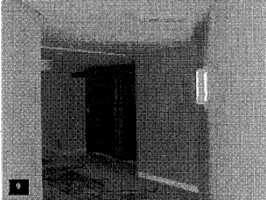
Tower Level T2 – View of a typical condominium entrance completed including doorbell, valance, finishes and hardware.
