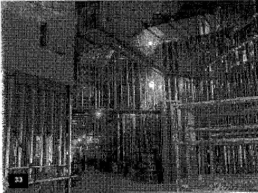
Podium Casino Level – View of the corridor adjacent to the Front Desk Support and the Coffee & Chocolate Boutique.
