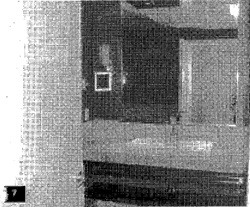
Tower Level T2 – View of a typical guestroom bathroom completed including; vanity top, sink, mirrors, valance and faucet.
