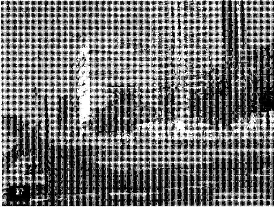
Garage/Convention Center – View of the southeast corner of the in process façade screening for the lower levels facing the residential towers and the completed EFIS façade facing the residential towers.
