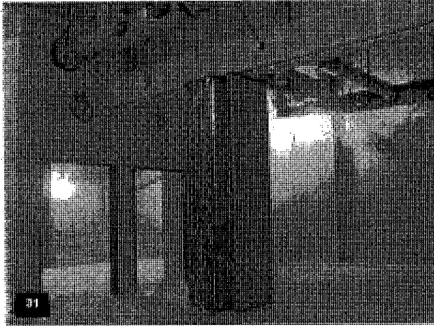
Garage/Convention Center – View of the installed operable partitions in the meeting rooms with the ceiling and MEP in process.
