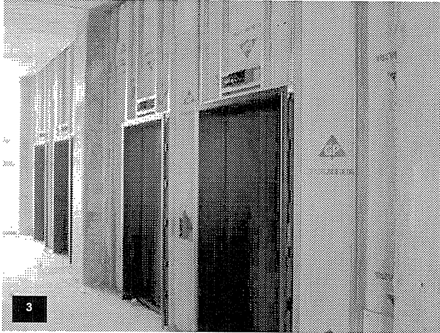
Tower Level T61 - View of the lobby area and the installed elevator doors.
