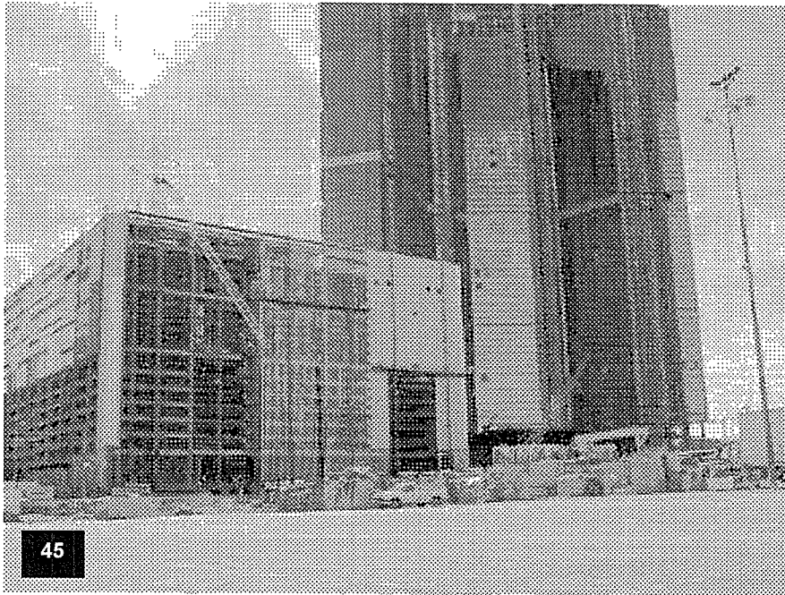
Garage/Convention Center – View of the north elevation of the garage façade with the exterior framing and installation in process.
