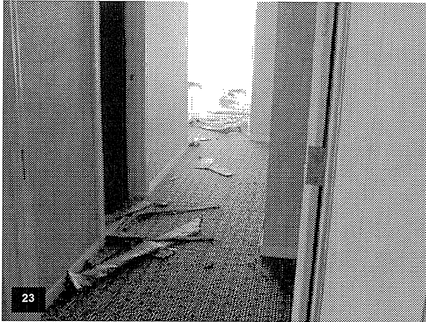
Tower Level T29 – View of a typical guestroom with the following completed: carpeting, base molding, wall covering and painting
