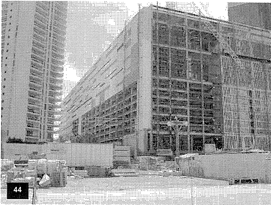
Garage/Convention Center – View of the northeast corner of the garage with the façade framing in process.
