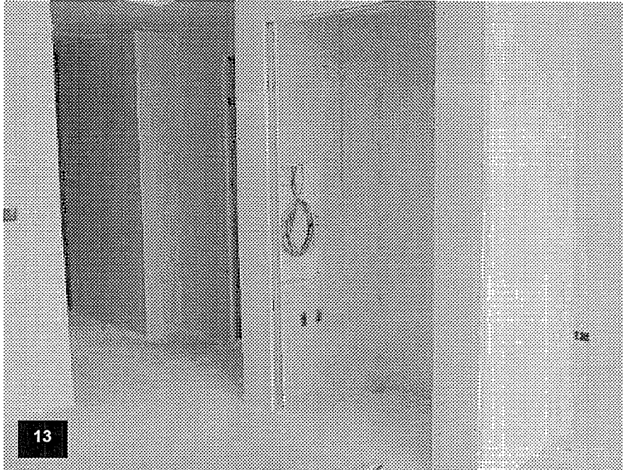
Tower Level T45 – View of a typical guestroom with the electrical rough-in completed and the gypsum board installed ready for taping and spackle.
