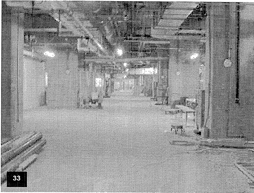
33 Retail Mechanical – View of the installation of the mechanical equipment in process.
