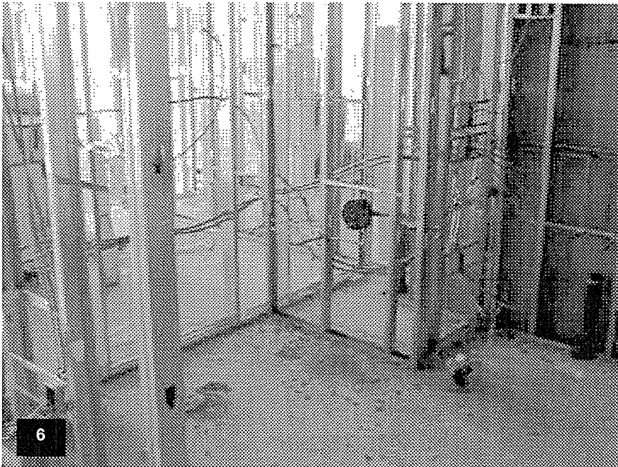
Tower Level T57 – View of a typical guestroom bathroom with the electrical and plumbing rough-in in process and the metal stud framing complete.
