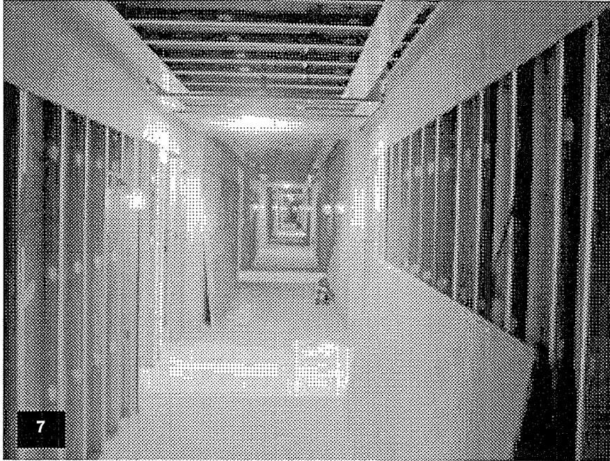
Tower Level T55 – View of the corridor with the metal stud framing complete and the gypsum board installation in process.
