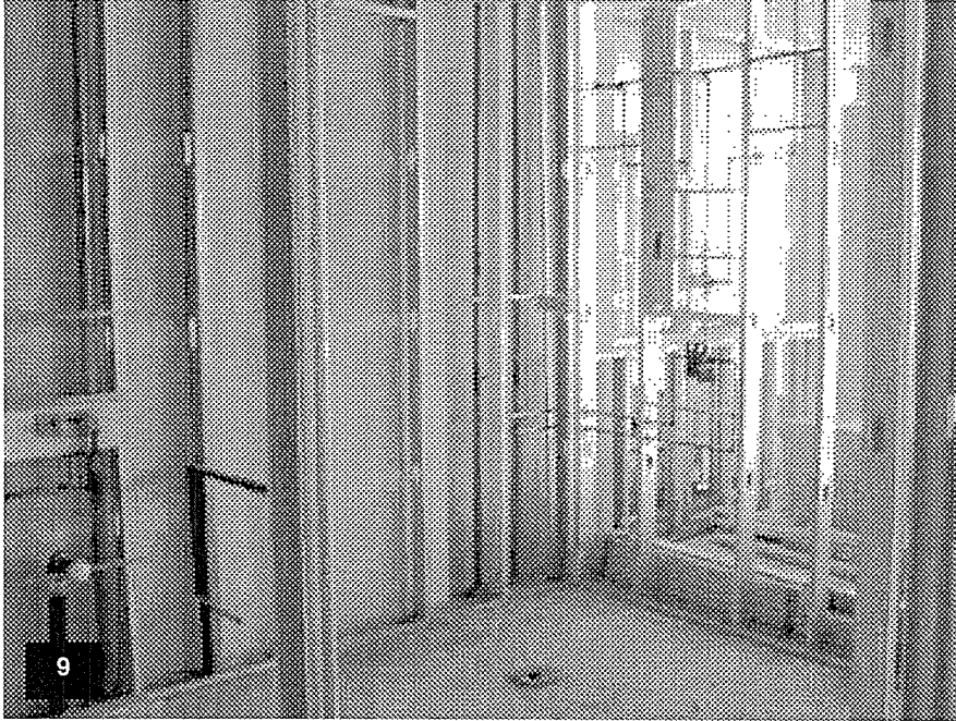
Tower Level T53 – View of a typical guestroom bathroom with the electrical and plumbing rough-in in process and the metal stud framing complete.
