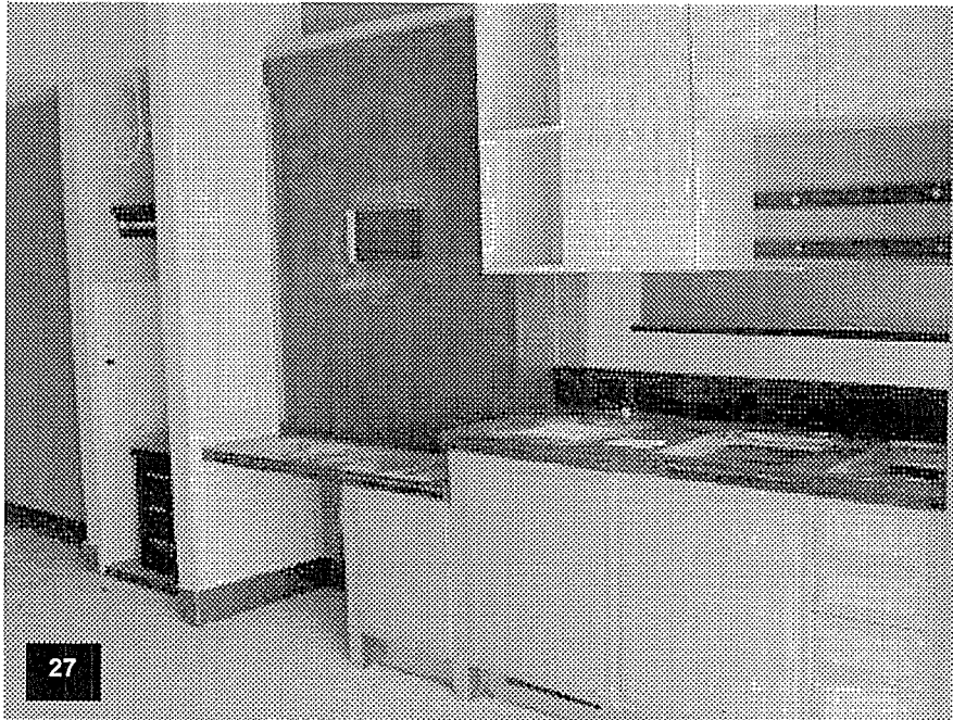
Tower Level T17 - View of a typical condo studio with the installation of the kitchen area in process including cabinets and countertop.
