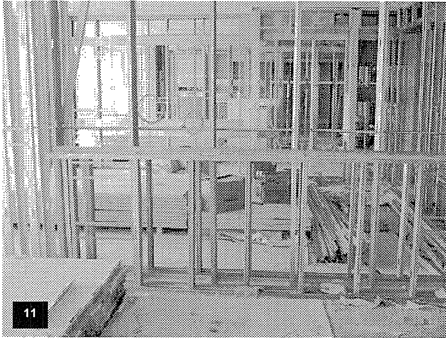
Tower Level T49 – View of a typical metal stud demising wall with a built-in shelf in process.
