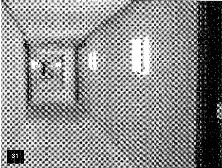
Tower Level T9 – View of the corridor with the installation of the wall sconces and wall covering completed.
