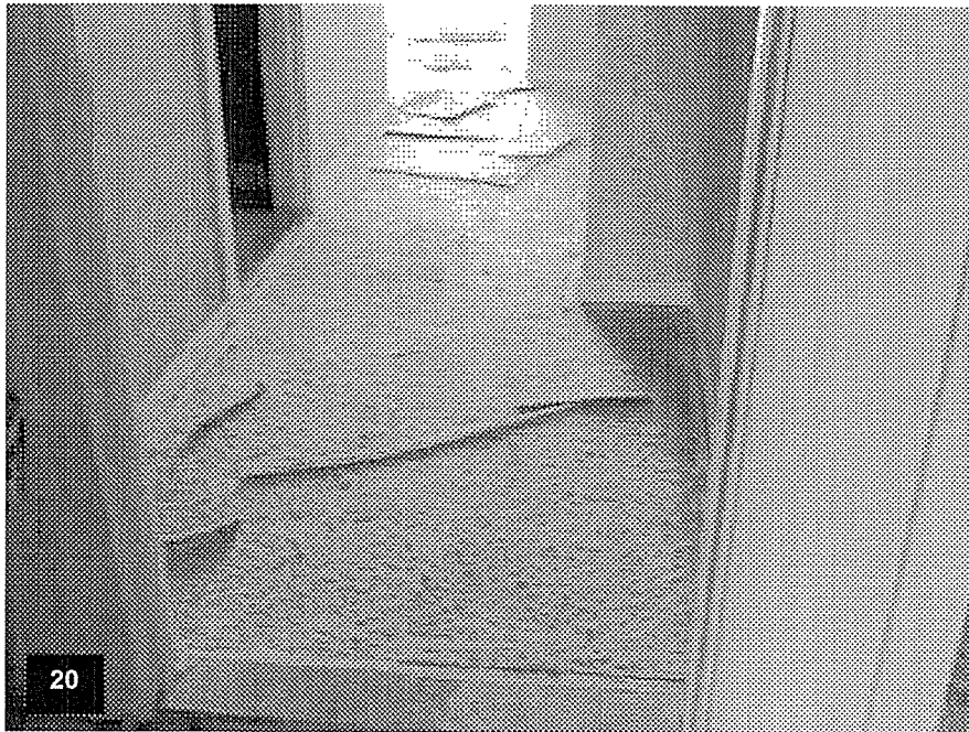
Tower Level T33 – View of a typical guestroom with the marble saddle and carpet tackless and padding installed.
