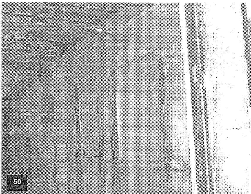
Tower level T-5 with corridor ceiling and wall framing and insulation complete, and drywall in process.
