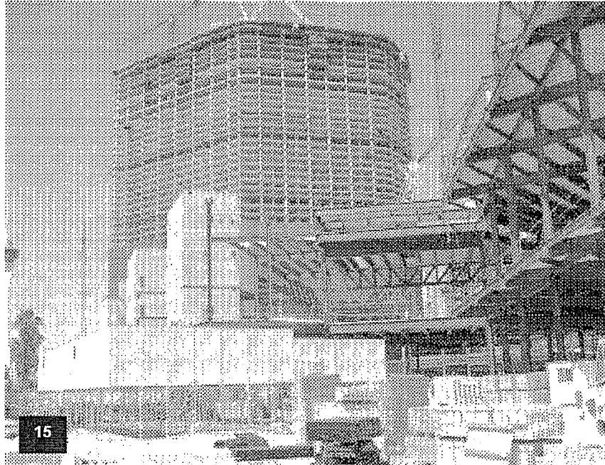
View of the south elevation of the Tower with the curtain wall system installed to Level T12
