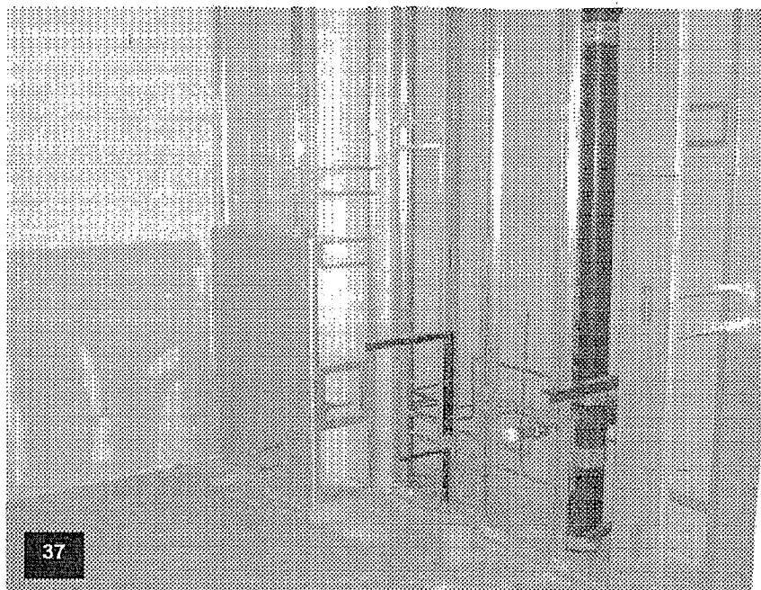
Tower level T-12 with wall framing complete, insulation and water proof dry wall in process, ceiling finish completed, plumbing risers and stub-outs in-place.
