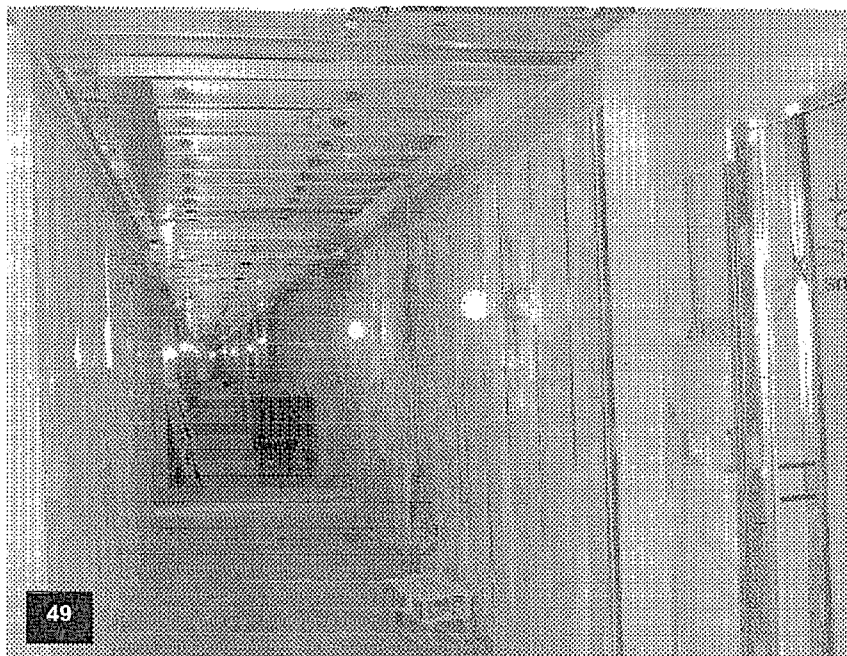
Tower level T-6 with corridor ceiling and wall framing and insulation complete.
