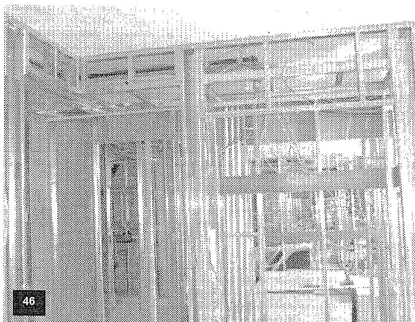
Tower level T-7 with wall framing complete, insulation and drywall in process, ceiling finish completed, and electrical conduit runs to outlet/switches in process and plumbing lines stubbed out for fixture connection.
