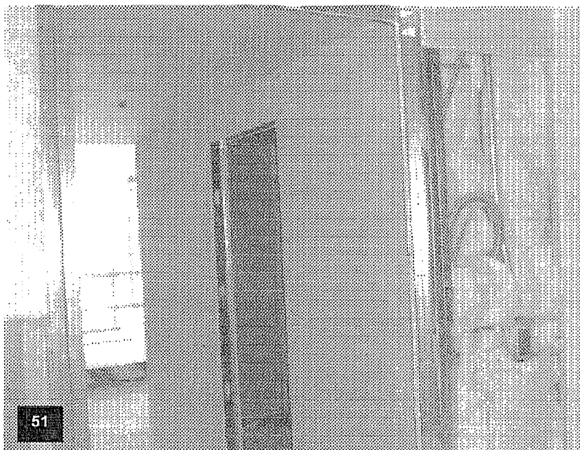
Tower level T-5 with wall framing and insulation complete, and drywall in process.
