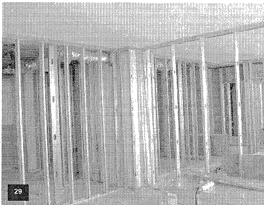
Tower Level T-20 with wall framing in process, ceiling finish completed, HVAC chase framed and drywalled, HVAC and plumbing riser/branch lines installation in place, and fire standpipe and branch line installed.
