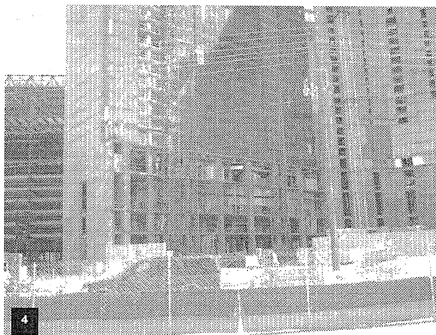
View of the tower's north elevation with the curtain wall system installed from Level T1 through T16.
