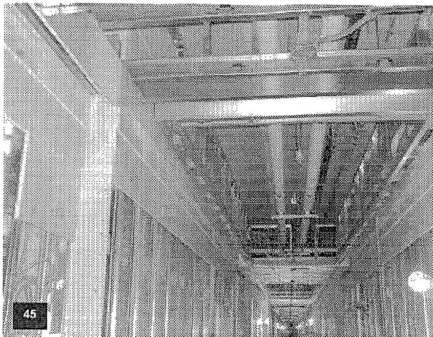
Tower level T-8 with sprinkler piping stubbed, and corridor ceiling framing in process.
