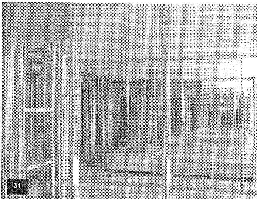
Tower Level T-18 with wall framing and drywall in process, door openings framed and ceiling finish completed.
