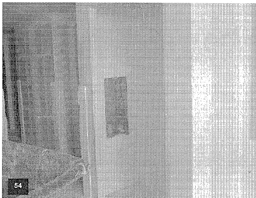
Tower level T-2 with suites framing, drywall, insulation, taping and spackling, electrical runs to the panel box complete and priming and painting of the walls in process.
