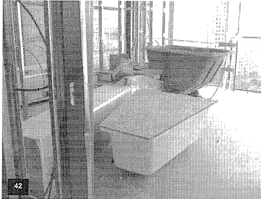
Tower level T-10 with bathroom soaking tub platforms framed/waterproofed and marble surround set and soaking tubs ready to be set. The curtain wall system (in the background) on the north elevation is installed to T16.
