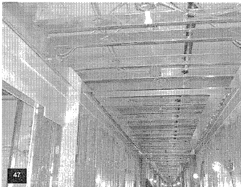
Tower level T-7 with sprinkler piping stubbed, and corridor ceiling framing completed.
