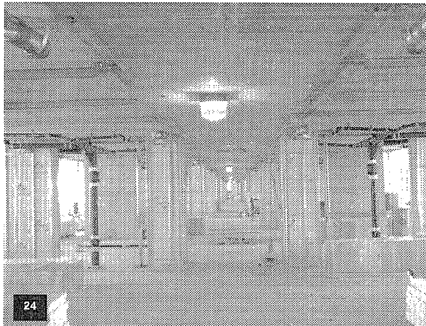
Tower Level T-25 with top track installed, HVAC chase framed and HVAC and plumbing riser/branch line installation in place.
