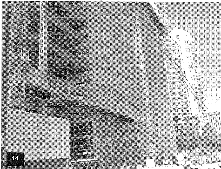
View of the south elevation of the Garage/Convention Center with 50% of the EIFS framing installed.
