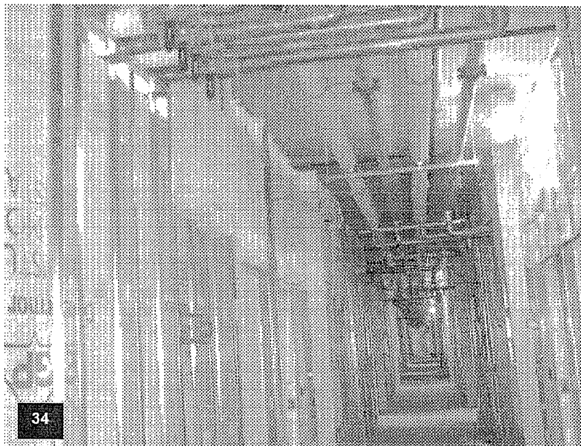
Tower Level T-15 with wall framing complete, insulation and drywall in process, ceiling finish completed, fire protection & MEP risers/branch lines installed.
