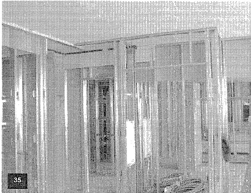
Tower Level T-14 with wall framing complete, insulation and drywall in process, ceiling finish completed, fire protection & MEP risers/branch lines installed and electrical panels in-place.
