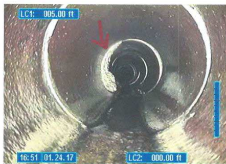
Figure 9: camera footage of the obstruction which prevented camera passage
