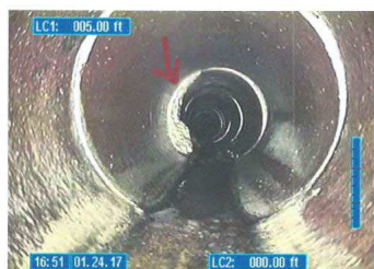
Figure 9: camera footage of the obstruction which prevented camera passage
