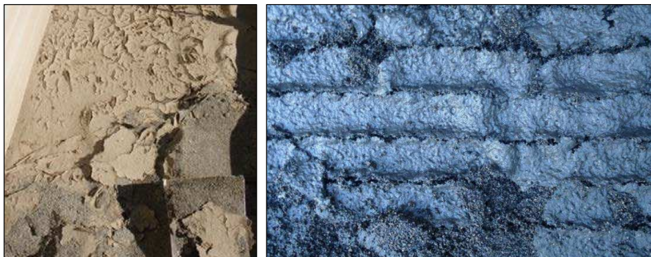
Figure 4. Accumulation of solids on the media bed surface
