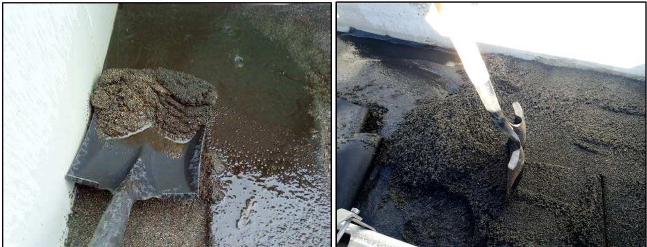
Figure 13. Surface cleaning (left) and measuring remaining inert media layer with a shovel (right).
