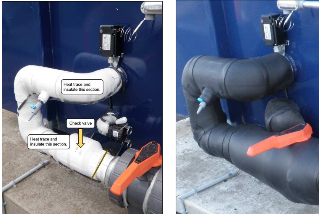
Figure 6. Aquip inlet line heat tracing (left) and Aquip inlet line insulation (right).
