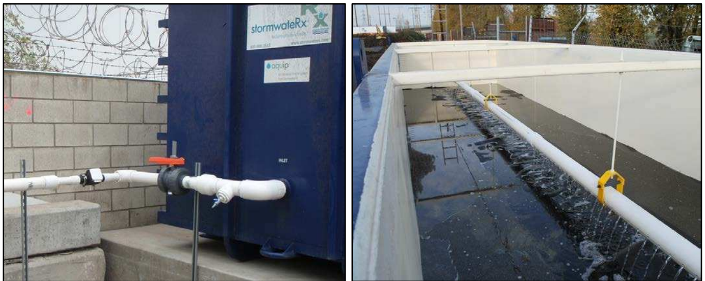
Figure 3. Inlet piping with flow meter (right); Uniform flow out the inlet distributor (left)
