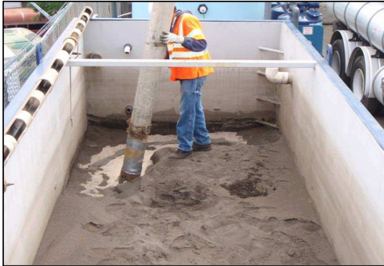
Figure 14. Vactor service removing the top layers of sand during a Seasonal Maintenance
