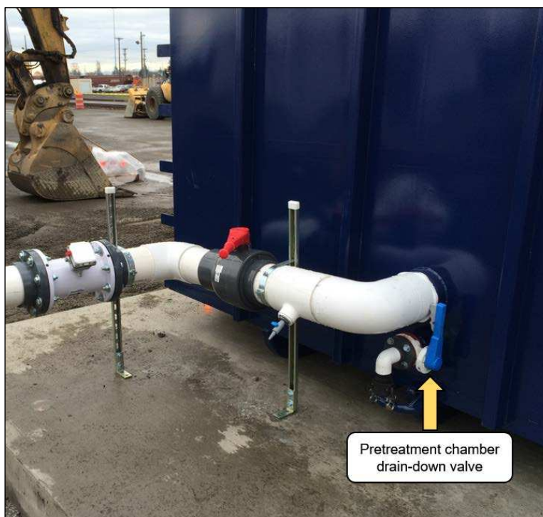
Figure 8. Pretreatment chamber drain-down valve
