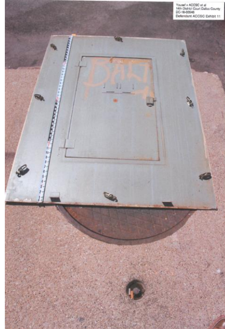
ACCSC Ex. 11 Inside of breaker panel cover detached from breaker box
